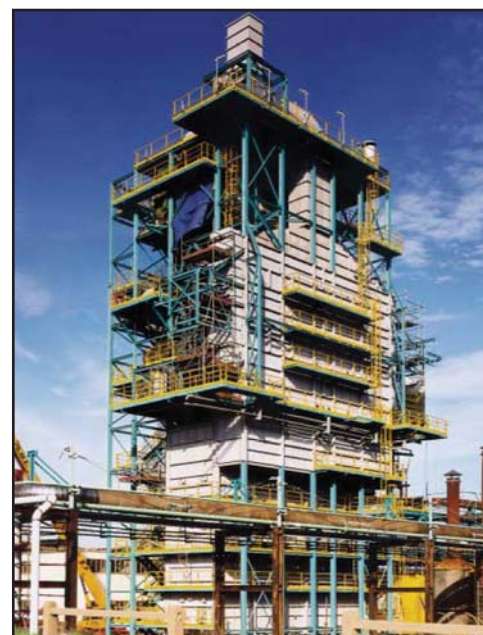
Ethylene Cracker Unit
